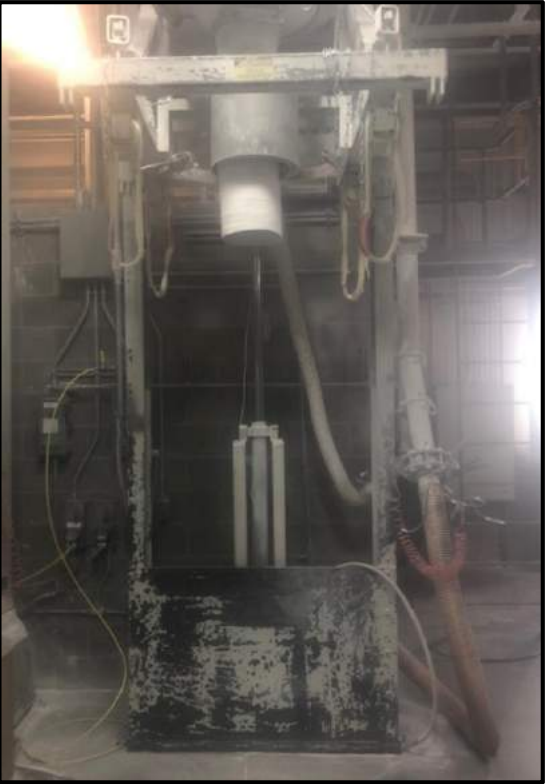
Existing Bag Fill Station. The Portable Drum Filler is manually position & connected to the Bag Filler.
